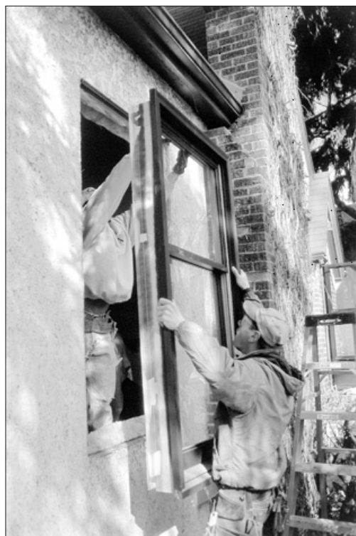
In the 65 DNL area, MAC has reduced home noise by installing windows, doors, air conditioning, and insulation.
