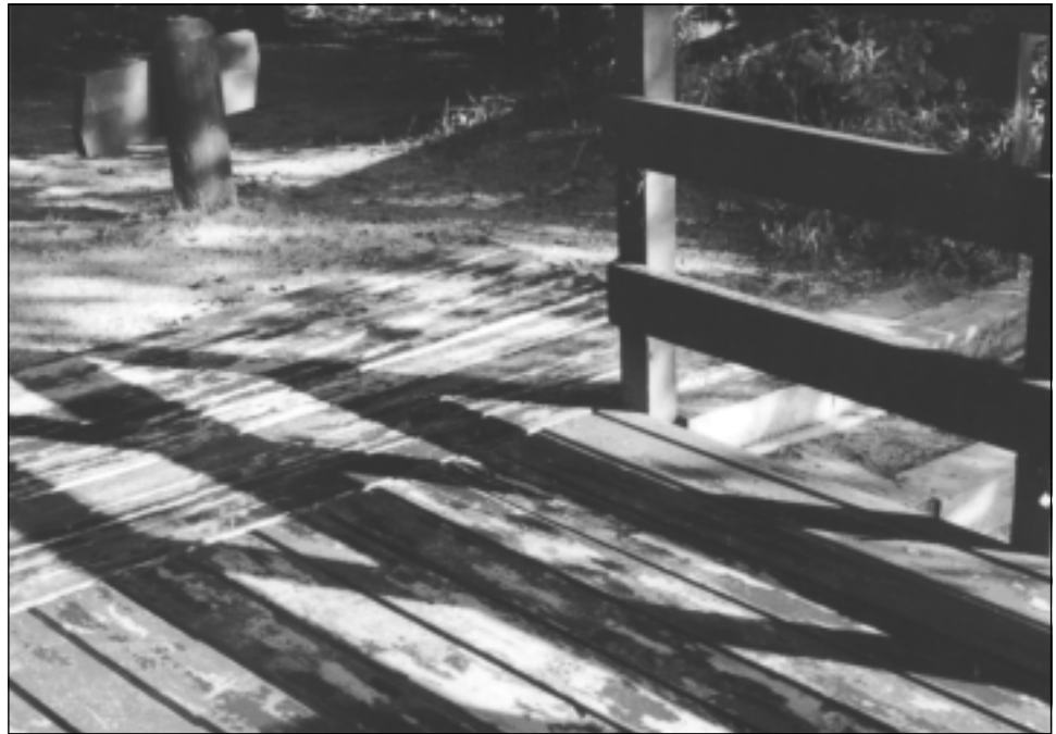
Painting is needed to protect decks and other wooden structures.
