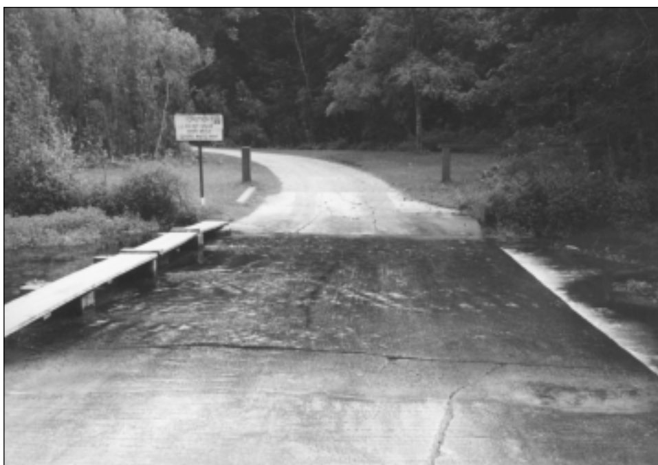
Replacement of the low-water crossing at Beaver Creek Valley is number 22 on the park capital improvement project list.
